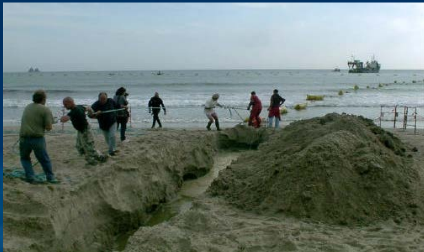
MEOC installation October 2001
